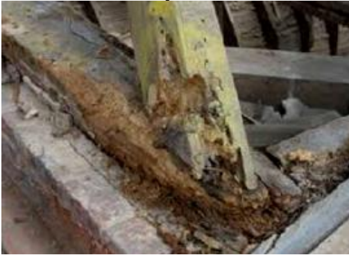
Figure 6: Brown rot Decay
