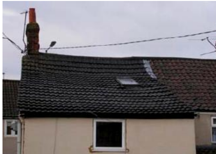
Figure 10: Sagging of roof
