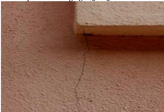
Figure 3: Crack between bay window corners
