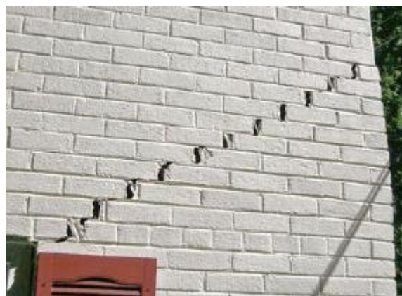
Figure 1: Foundation wall cracks
