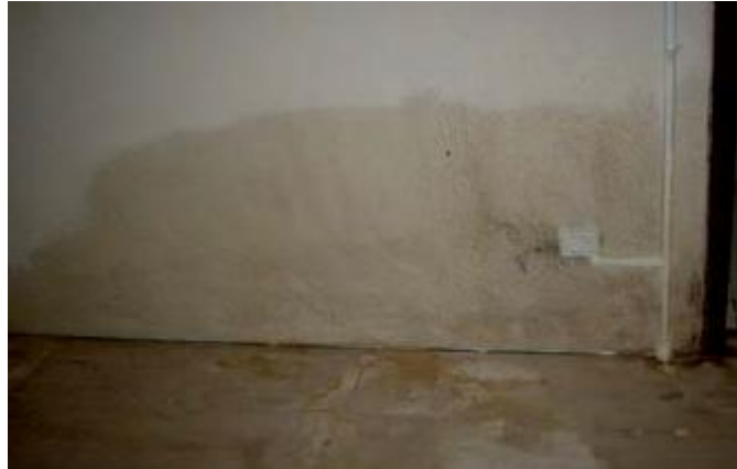
Figure 5: Rising dampness problem
