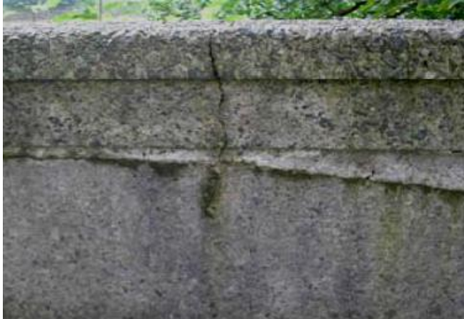
Figure 2: Cracks at the centre of panel
