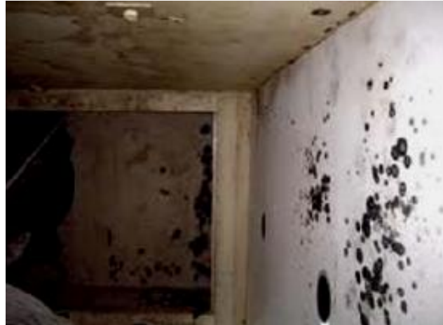
Figure 9: Fungi on internal wall
