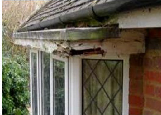
Figure 7: Timber decay of Flat roof
